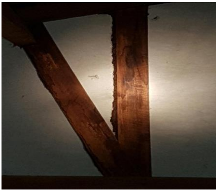
Workings in the roof space with no structural damage noted in the accessible areas checked.
