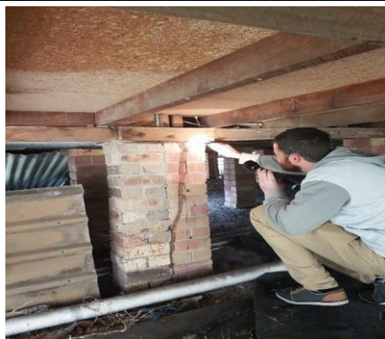
Visible evidence of subterranean termite workings and/or damage was found at the time of inspection. It was in, but not necessarily limited to the following location(s)piers and subfloor up to the ceiling.
