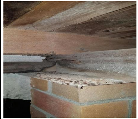
Visible evidence of subterranean termite workings and/or damage was found at the time of inspection. It was in, but not necessarily limited to the following location(s) subfloor bearers have damage and have weakened due to the floor loads. Recommend builder repair or support the bearers where damage occurred.
