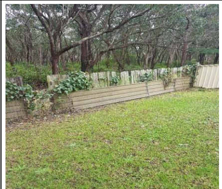
Termite damage and workings to Fences was detected, notably those in direct contact with the ground and also in some cross-rails and posts.
