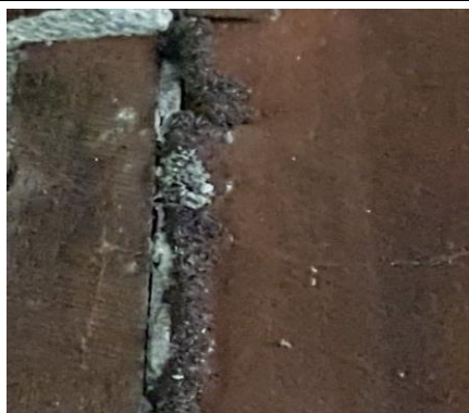
Visible evidence of subterranean termite workings and/or damage was found at the time of inspection. It was in, but not necessarily limited to the following location(s)the garage.
