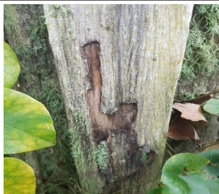
Termite damage and workings to Fences was detected, notably those in direct contact with the ground and also in some cross-rails and posts.
